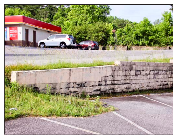
The city will soon be installing a guardrail here at Jackson Street to protect against cars that accidentally roll downhill from Circle K from time to time. Photo by Shawn Jarrard
